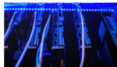
Liquid immersion cooling Ideal for 50-200 kW Rack load
